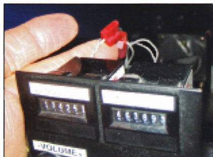
A close look at the connection made at the meters.
