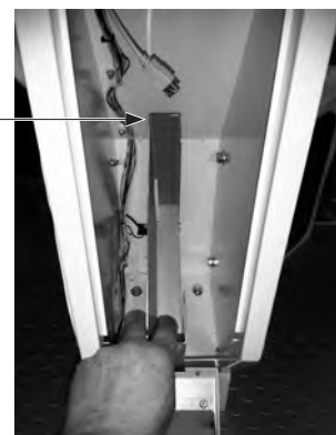
Lift Ticket Holder at the rear before removal.
